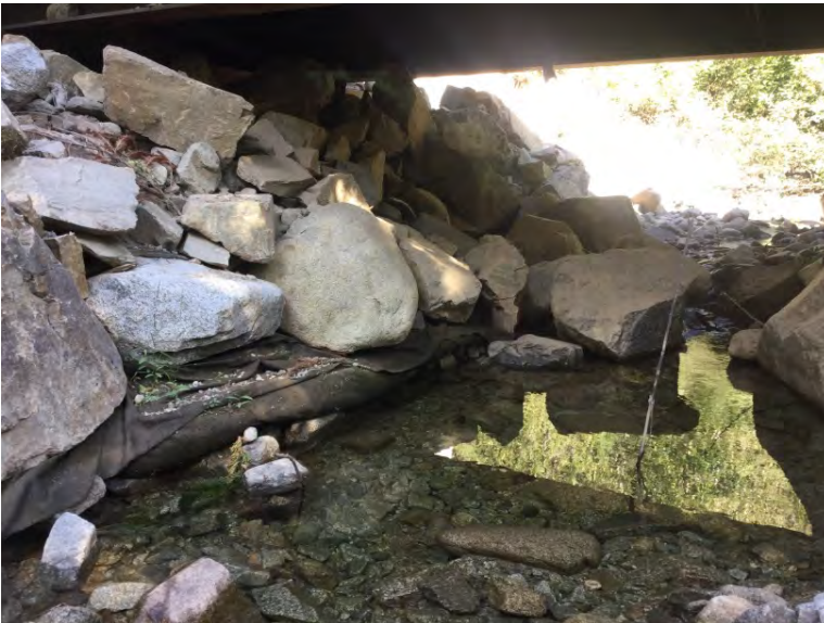
Right bank riprap scour and failure
